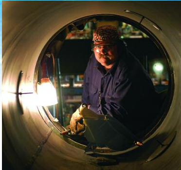
Welder Stephen R. Hardee, a native of Lenoir, N.C., is working on the shaft tunnel.
