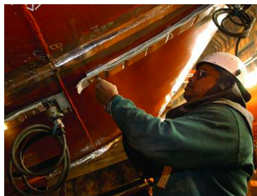
Welder David G. Darnell is a native of Lumberton, N.C. He is attaching a heater bar to the hull of North Carolina to prepare to weld hull units.
