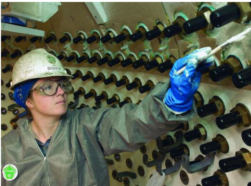
Insulator Cassidy E. Bishop, originally from Washington, N.C., applies insulation in the sonar sphere.
