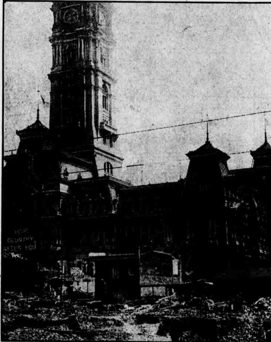
THE DEMOLITION FOR THE PARKWAY GOES ON, AS THIS VIEW FROM ARCH STREET ATTESTS
